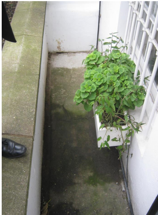
Front elevation with No.12 on right (top) and existing front lightwell (bottom).
